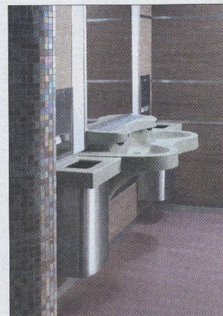
Proximity-sensing faucets, light-operated by photovoltaic cells, reduce water consumption and electricity use, as well as help keep batteries out of landfills.
