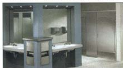
Good design and durability can go hand-in-hand, as this stylish public washroom amply illustrates.
