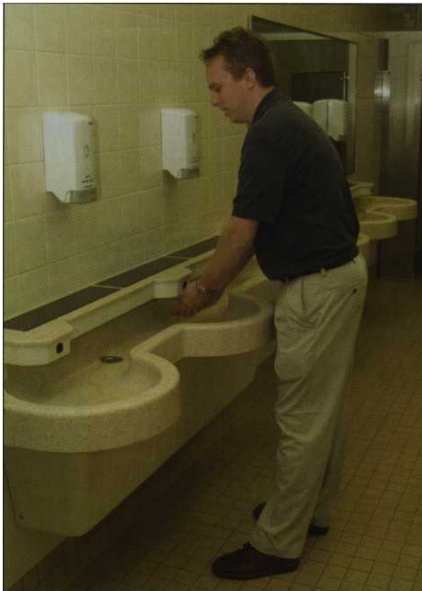
This Wal-Mart restroom utilizes solid surface lavatory systems, which are durable and easy to keep clean. It also has light-activated sensors for soap and water.
